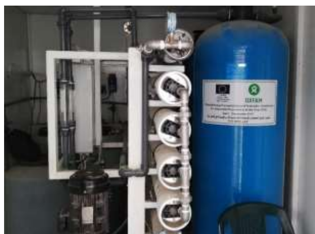
Figure 8 – Al Amal Solar RO system, Gaza
