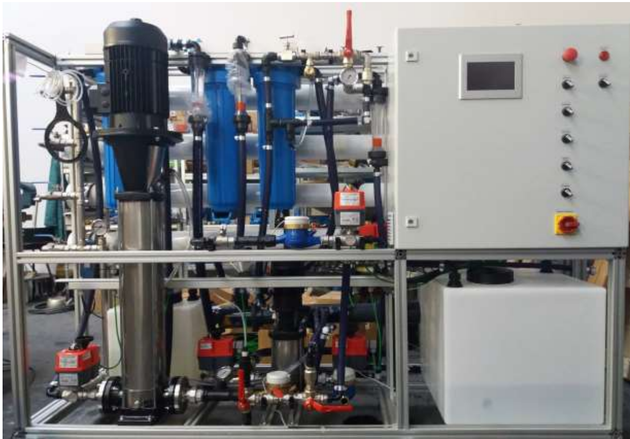
Figure 9 – Oxfam Somalia RO system components (Boreal Light)
