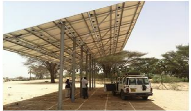
Fig 11: Pole mounted structure in Turkana, Kenya
