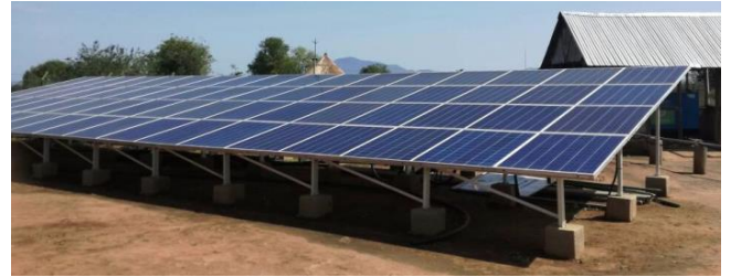
Fig 10: Ground mounted support structure in Rhino Camp, Uganda
