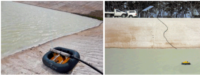
Fig 9: Submersible pump installed on a floating pontoon
