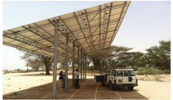
Fig 11: Pole mounted structure in Turkana, Kenya
