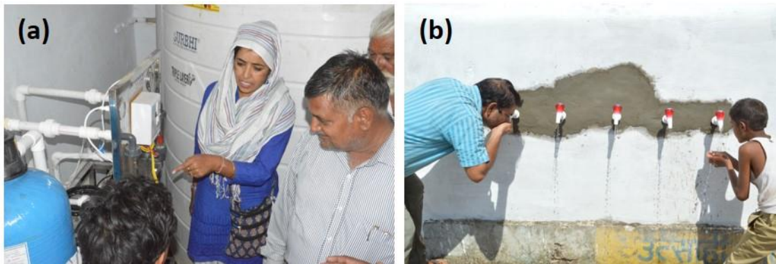
Figure 17: The Barefoot College's solar-powered RO unit in a village near Sambhar Salt Lake, Rajasthan, India: (a) local woman explaining the water purification process; (b) a village drinking fountain being supplied by PV-RO.
