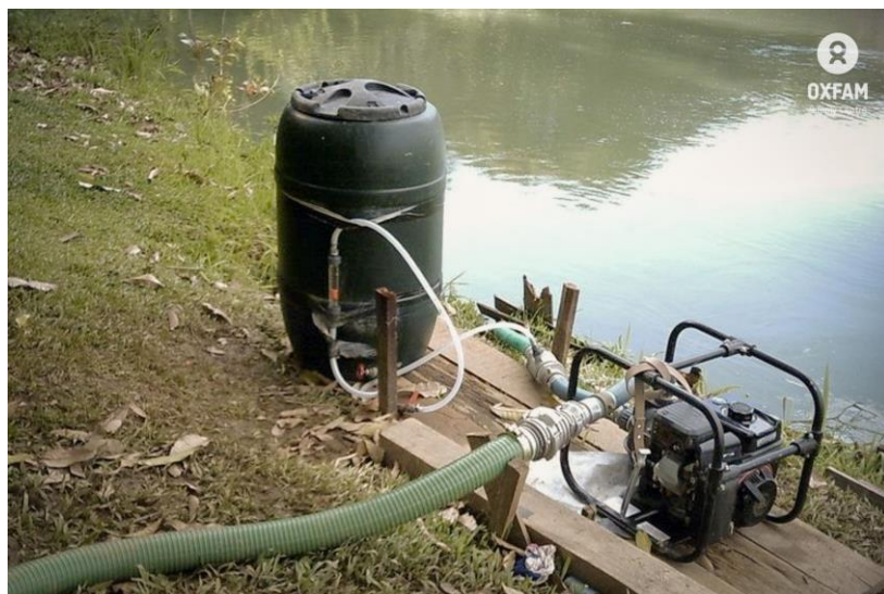
Figure 6 – Example of suction side dosing
