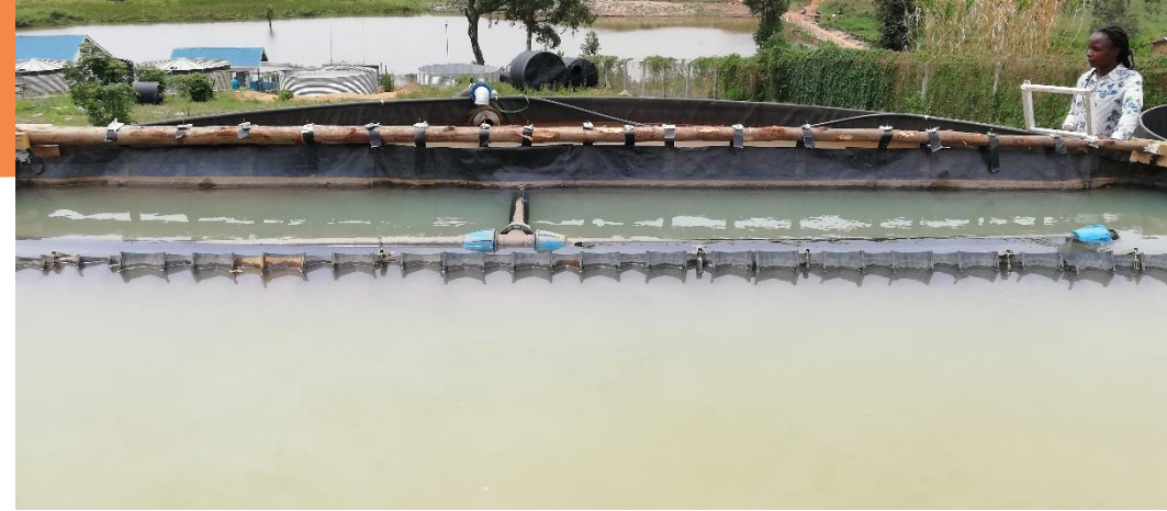
Risk of overtopping lamella (and short circuiting) if inflow is too high
